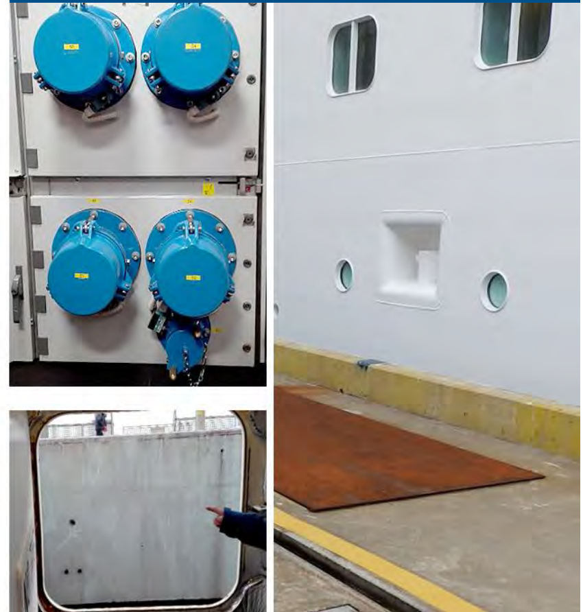
Ship's hatch / Control Cabinet
